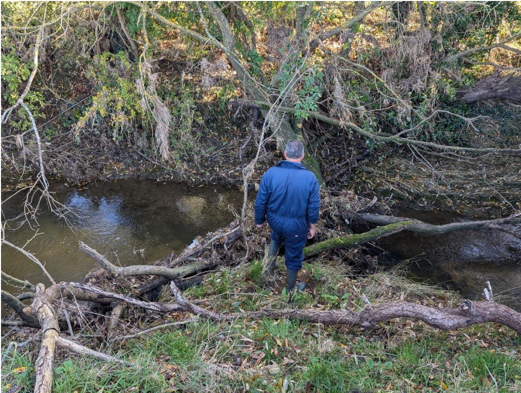
Figure 19: Obstruction H during subsequent low water levels in Grendon Brook with resident for scale showing size and extent of blockage as well as difference in water levels up and down stream of obstruction, illustrating its effect at holding back water. © C. Dow
