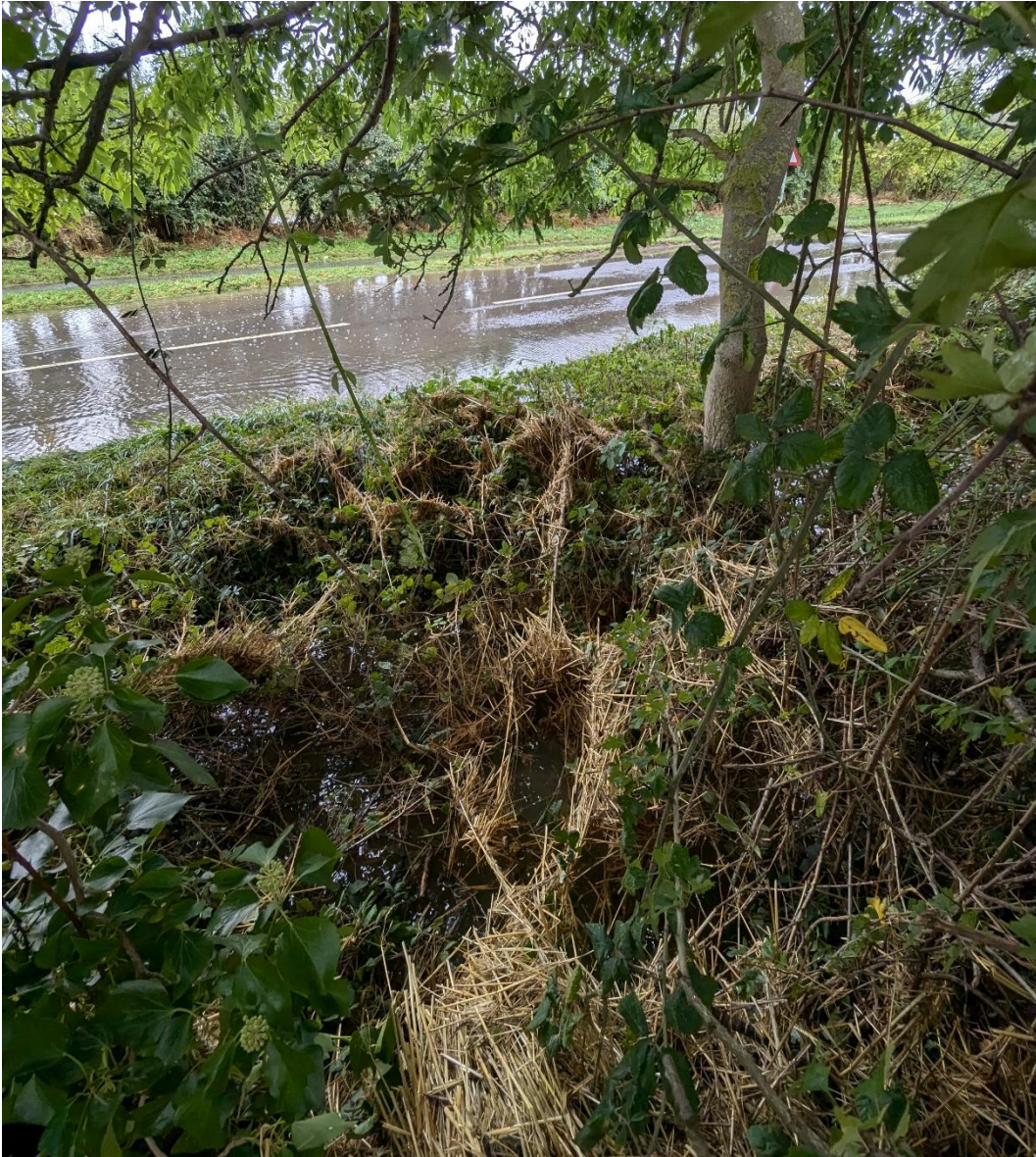
Figure 21: Obstruction K showing overgrown and filled in condition of ditch along Main Road adjacent to Flexlands field running to Grendon Brook. Note mature tree growing in centre of ditch. © C. Dow
