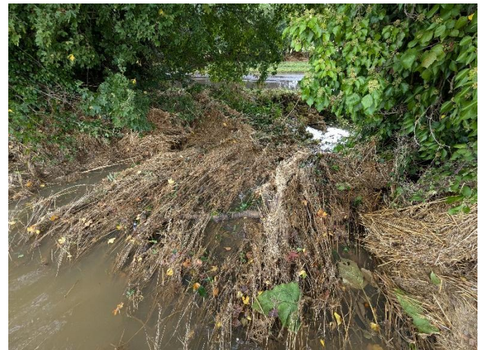
Figure 16: Example of a breached detritus dam from Flexlands onto Main Road at Obstruction K. © C. Dow
